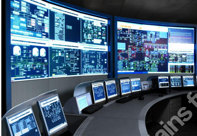
Figure 1. ICS Control Center displays (prohest, 2014).
