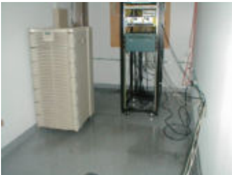
More water damage in the server storage space.
