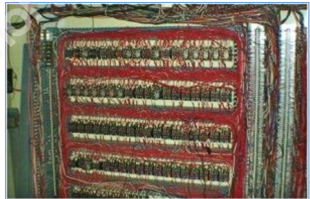
Figure 7 Picture of Factory Relay Rack ( http://www.blog.beldensolutions.com/wp-content/uploads/Old-Relay-System-300x195.jpg )
