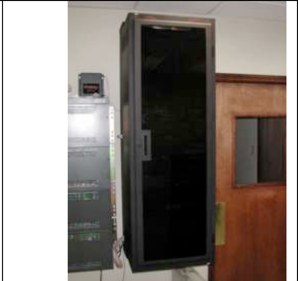
Figure 3.4 Cabinet housing firewall
